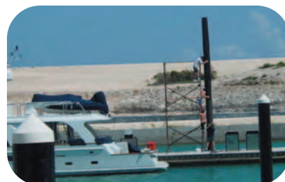
Heat Shrinkable tubing being installed over the existing pilings before being shrunk in place.
