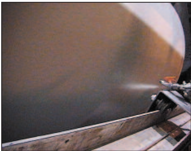
Fluoro-Coat 200 applied to a dryer in an eight-hour outage provides a release surface for years.
